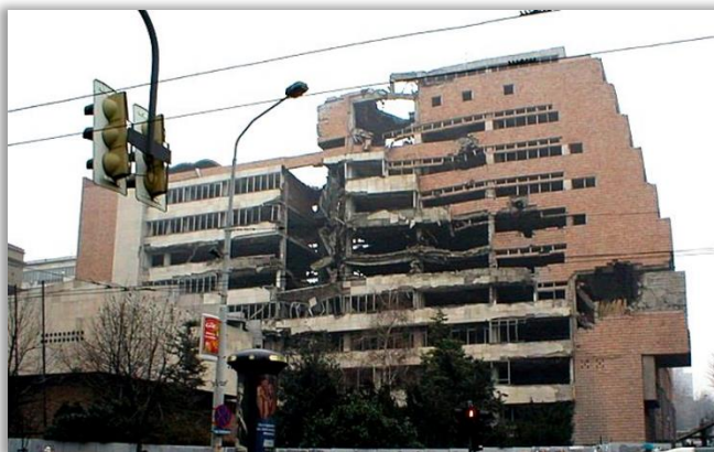
Fig. 16: Former Serbian Ministry of Defence building destroyed by NATO attacks in 1999, (Source: Wikipedia)
